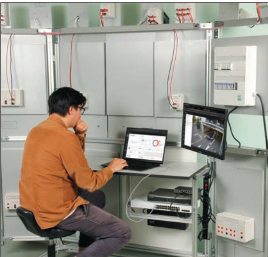
Rear view of the entire supervisory station
