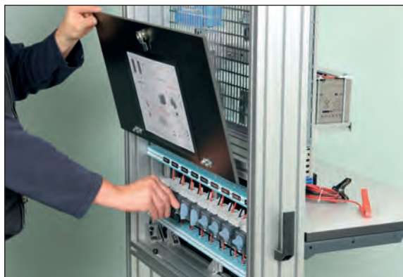
Flap for access to the switches
