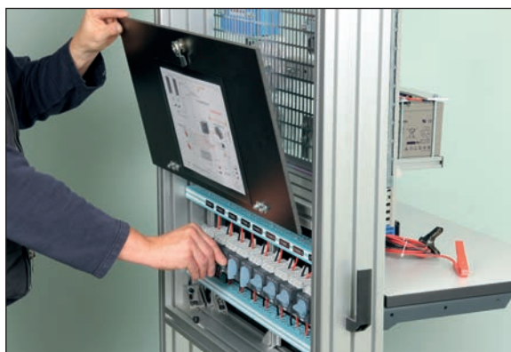
Flap for access to the switches
