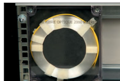
fiber optic coil of 2 km
