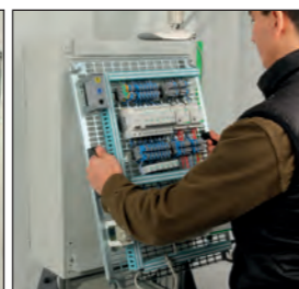
Grid support at the back of the box allowing the wiring of the grid before it is used in the cabinet.
