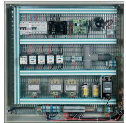
Inside view of the cabinet
