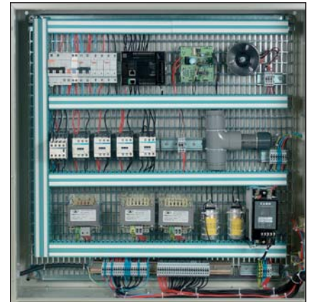
Inside view of the cabinet
